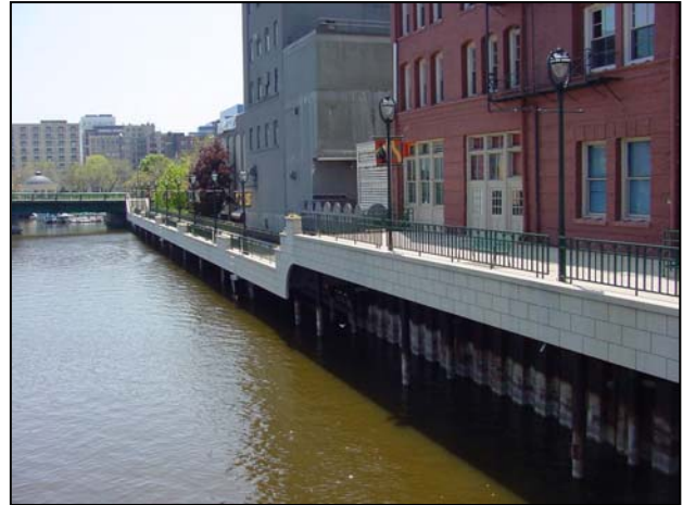
The cantilever technique (with pilings) has been successfully implemented in other Wisconsin communities.
